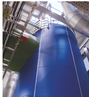
Water heating boiler
