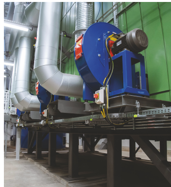
Biomass furnace PKS-15
